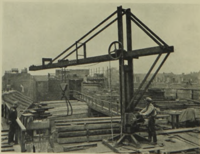
LIGHT ROOF CRANE.
