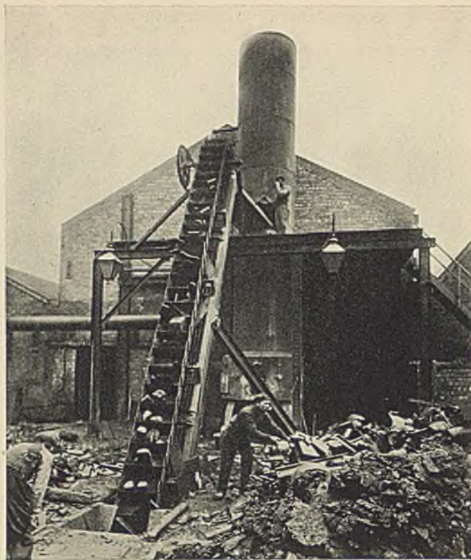
18-INCH BUCKET ELEVATOR FEEDING FOUNDRY CUPOLA.
