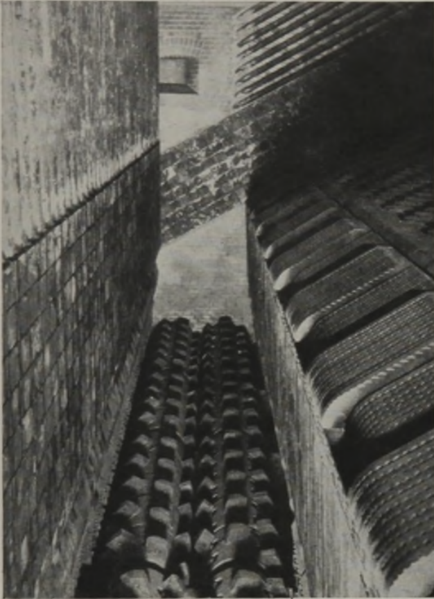
FIG. 80.—View of lower end of Taylor stoker and of ashpit.
