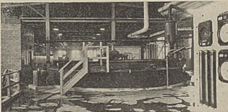
Below—Cell liquor containing salt and caustic is transferred to this large tank for crystallization of the salt. The caustic is then sent to evaporators, to make desired shipping strength
