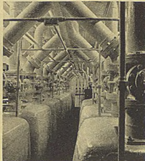
9 These manifolds connect the high-vacuum dryers to the roughing and diffusion pumps
