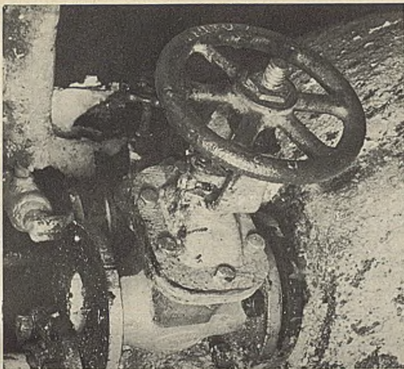
Corrosion often occurs in dangerous and inaccessible places as in this pipeline in a petroleum resin plant which had to be replaced with high Ni-Cr-Mo alloy steel after a costly failure of valve and fittings
