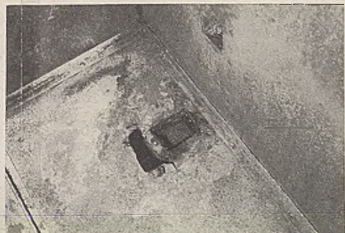
Inside of the dried grain bins and ducts steel plate is badly damaged, probably as a result of a combination of corrosion and erosion. Raw-mash proves equally corrosive
