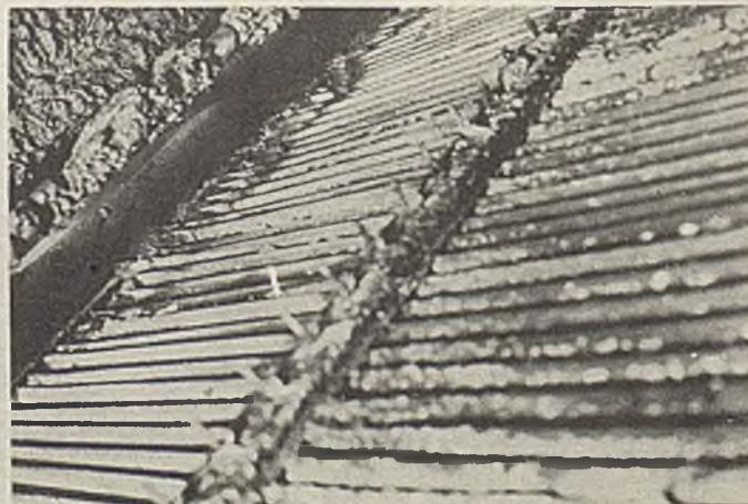
Aluminum baffle plates in the dust collectors of a grain drying unit in a whisky distillery now converted to the production of industrial alcohol were seriously corroded
