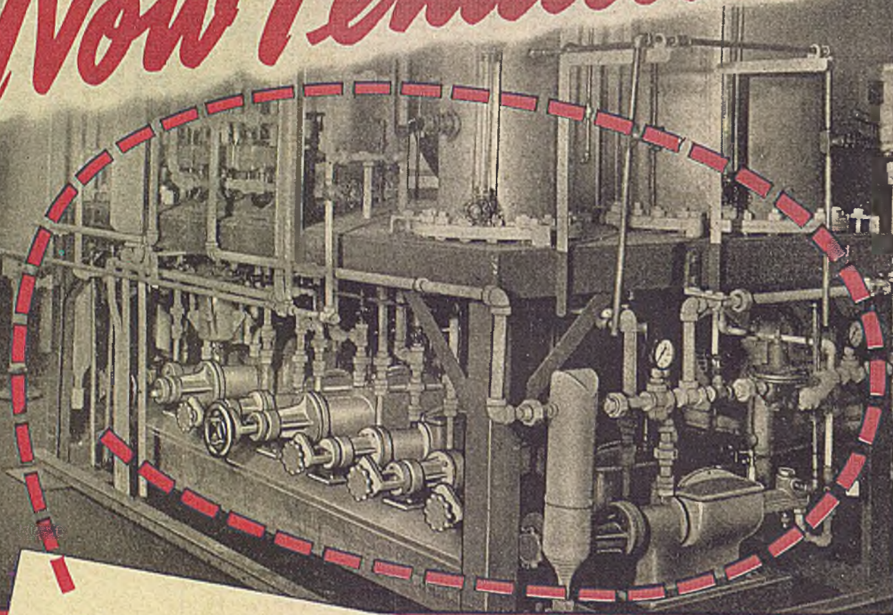
Compact battery of %PROPORTIONERS% Treat-O-Units used by Commercial Solvents Corp. in producing Penicillin.
