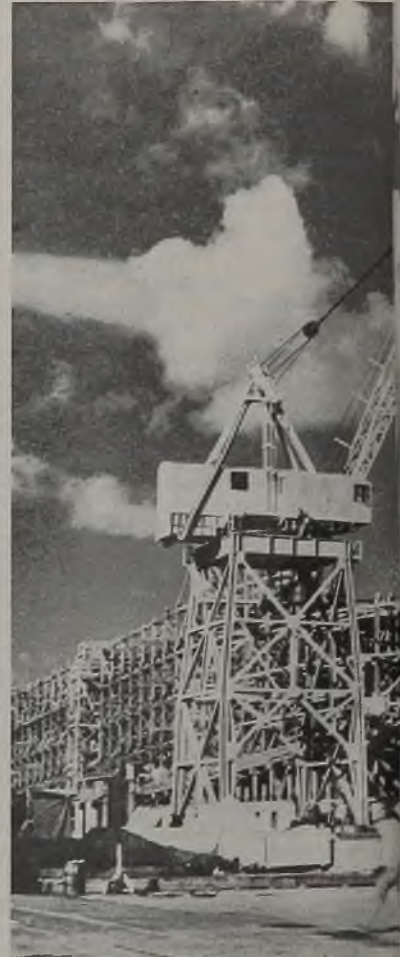
Forepeak section of a cargo ship is hoisted into place at the yards of the California Shipbuilding Corp., above. NEA photos, except where otherwise credited
