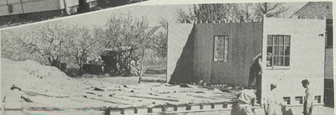
At left is a four-room house, prefabricated and constructed to be erected in a day. Cost is less than $4000. Below the house at start of erection is shown
