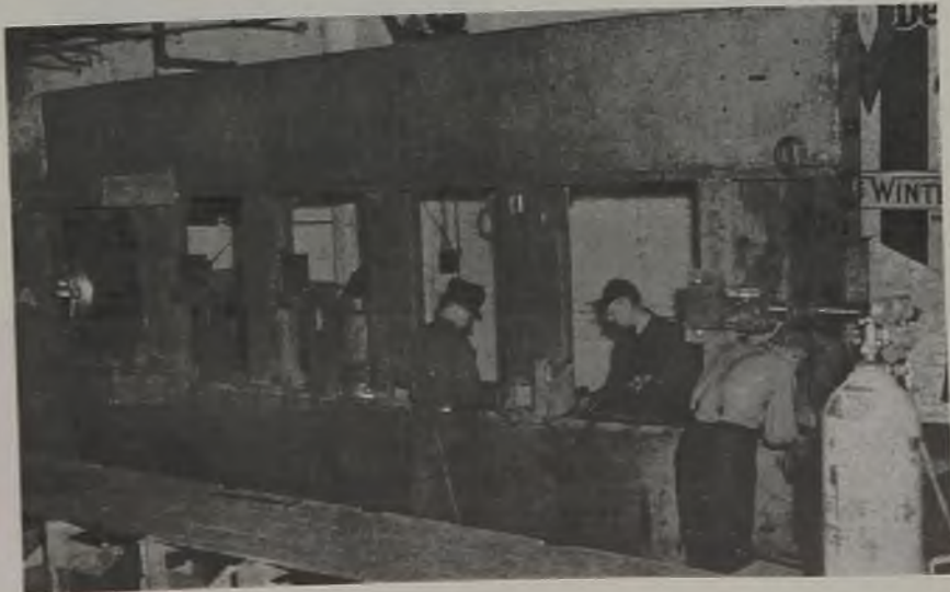
(Left) — Slagging positioner used to remove weld spatter and slag are removed. This is same type positioner used for finish welding
