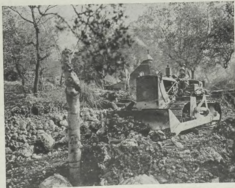
BULLDOZER: Caterpillar diesel tractor with LaPlant-Choate bulldozer knocks down an erosion wall along the mountain road between San Pietro and San Vittore to allow two-way traffic to and from the front in Italy. Signal Corps photo
