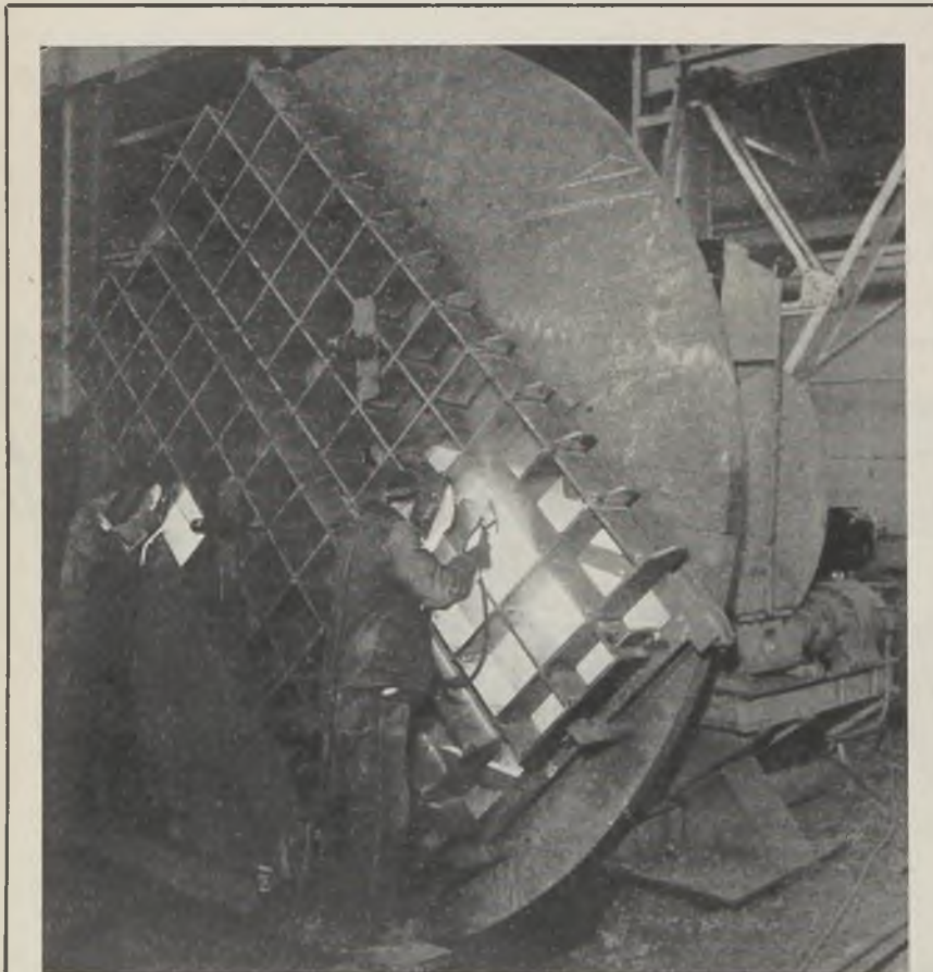
A-C WELDING DOES IT —A welding speed about 20 per cent higher than was possible with direct-current welding is reported by Mississippi Valley Structural Steel Co. as a result of switching to a 500-ampere alternating-current arc welding transformer to fabricate these heavy steel gratings. Magnetic disturbance to the arc and consequent undercutting, experienced with the direct-current method, has disappeared and operators are able to deposit weld metal the full length of the joints on the inside of each cell-shaped opening. This also permits higher current and, in turn, more speed. Electrodes used are General Electric type W-24
