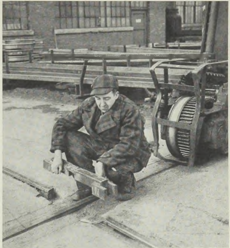
PROBLEM'S ANSWER: Portable railroad track inserts, placed in position over the gantry yard crane rail, opened an additional entrance to the Locomotive division shop at General Electric Co.'s Erie Works. Because the driving gear and wheel of the crane are practically the same diameter, a regular crossover was not satisfactory since the driving gear would hit the railroad track each time a crossing was attempted
