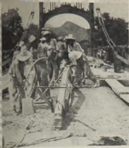
Native road workers leveling concrete on Guatemalan bridge, part of Inter-American highway. Page 70
