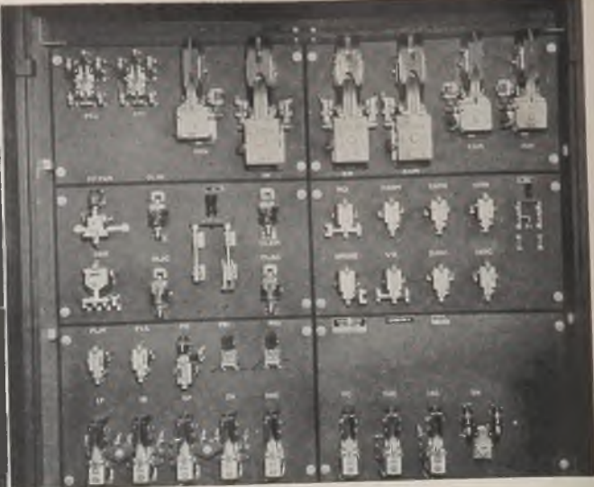
Fig. 15 (Above left)—A-C drawbench control panel for 200/100-horsepower main drive and miscellaneous auxiliaries
