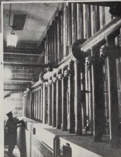
Fig. 1 (Top)—Cylinders containing 50 pounds of liquefied carbon dioxide under 850 pounds per square inch pressure at 70 degrees Fahr. are manifolded in five frames of 56 cylinders each. Released in the lines and controlled by directional valves, gas rushes to the burning area and is completely distributed within 1 minute
