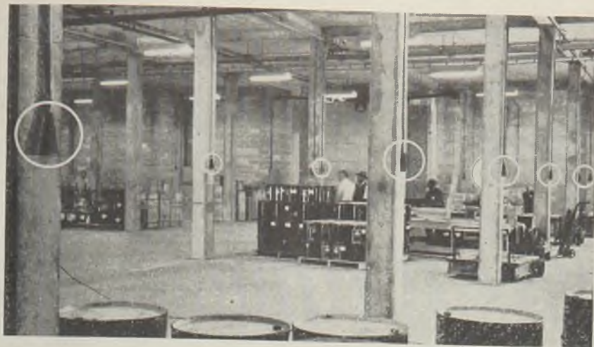
Fig. 3—One of the storage spaces for highly inflammable materials, showing multiple discharge nozzles (encircled) arranged in sprinkler fashion on columns and against wall. These deliver in less than 30 seconds a concentration of fire-smothering gas throughout the room
