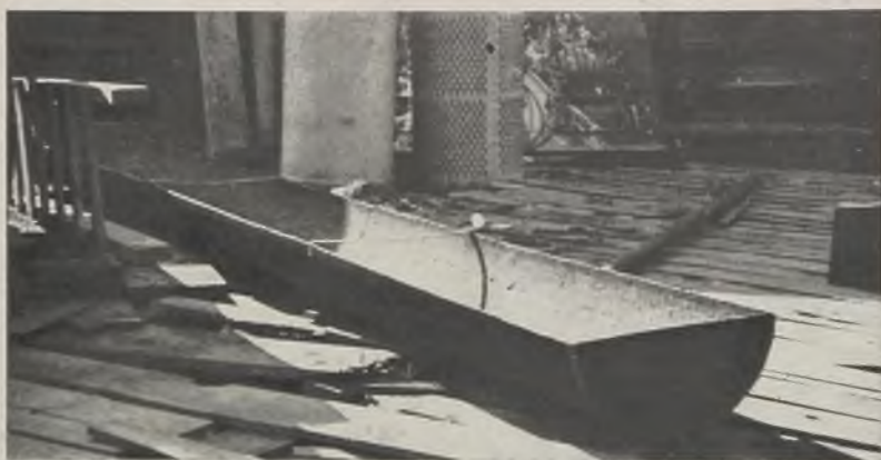
SHEEP FEEDING TROUGHS: Steel feeding troughs are being fabricated by the Bernstein Bros. Lumber & Supply Co., Pueblo, Colo., by cutting 18-inch pipe lengthwise in half so that each length of pipe will make two troughs. The ends are closed by welding in steel half circles and a few strips across the top provide rigid support. An unusually good market is reported for the troughs which sell at $1 per running foot
