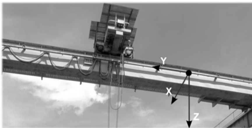
Fig. 8. Axis of measurement system for test object (Experimental research crane – OBRDiUT "Detrans" in Bytom)
