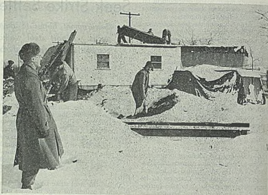
Workmen erect prefabricated houses on the site of a wartime Army camp on the northern edge of Chicago. These units will be used by returning veterans. Some of the houses were completed just before Christmas. NEA photo
