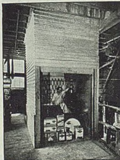
Note this factory installation in which hoistway is not against any outside wall, and with two gates giving access to different levels.
