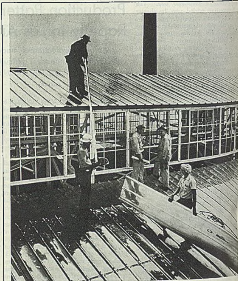
ALUMINUM ROOF: This aluminum roof recently was installed over the cast house at Reynolds Metals Co. plant in Louisville, Ky. Tests have shown the 24S-T pure clad alloy 0.032-gage sheets will wear well and resist the corrosion by cast house fumes
