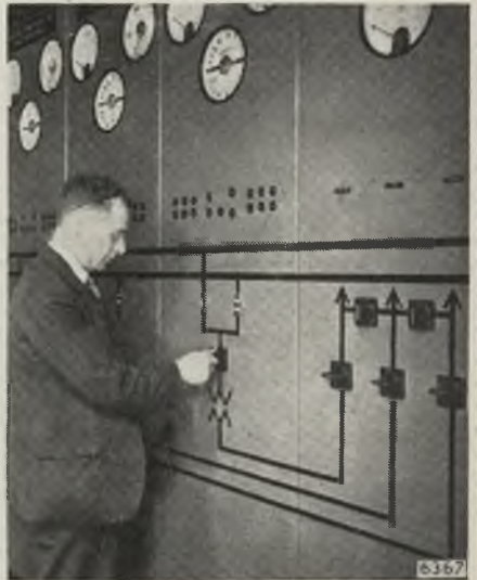
Fig. 4. —Portion of mimic diagram on control board, incorporating the type FLC switch
