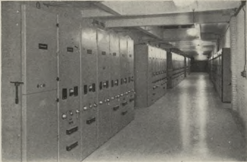
3.3 kV English Electric air-break switchgear
