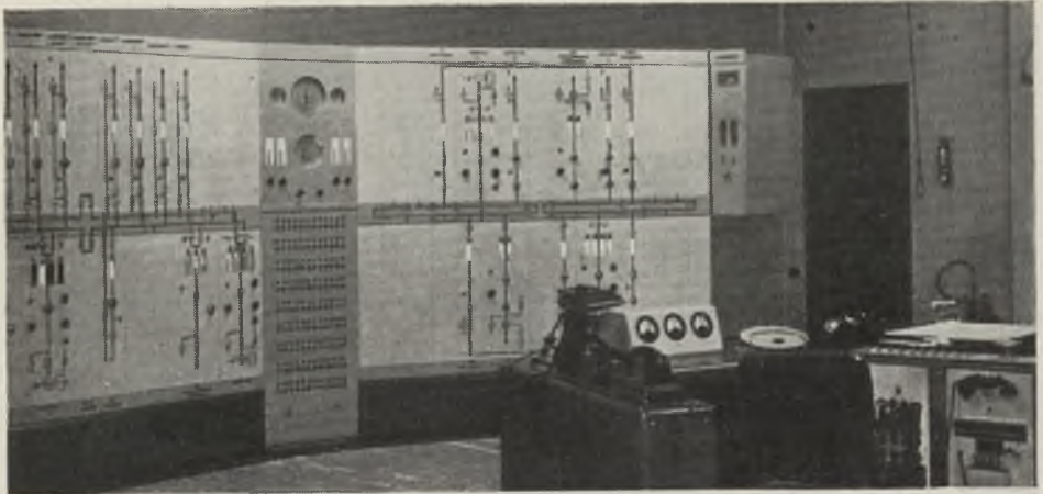
The main panel in the control room
