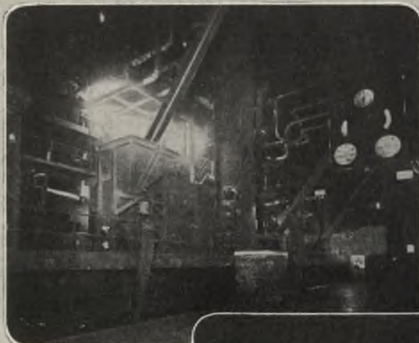
Left:—View of part of the pulverised fuel boiler platform at Littlebrook
