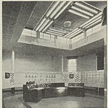
The control room. A unique feature is that the panels are supported on columns
