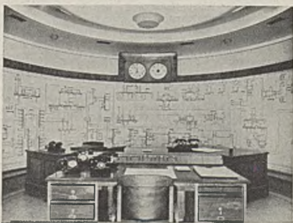
Area switching room
