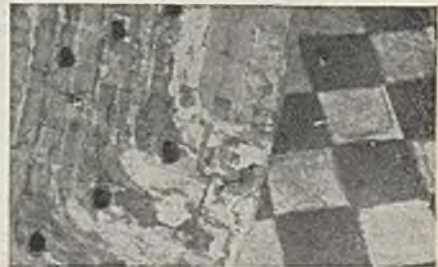
Fig. 4.—Exciter end of rotor, showing where portion of top turn has welded itself to end cap, also where some parts of bonding strip have become welded to cap
