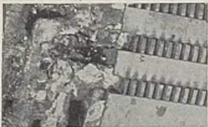
Fig. 5.—Exciter end of rotor, showing position of earth fault and burning of part of core as the result of arcing; also where portion of top turn is missing
