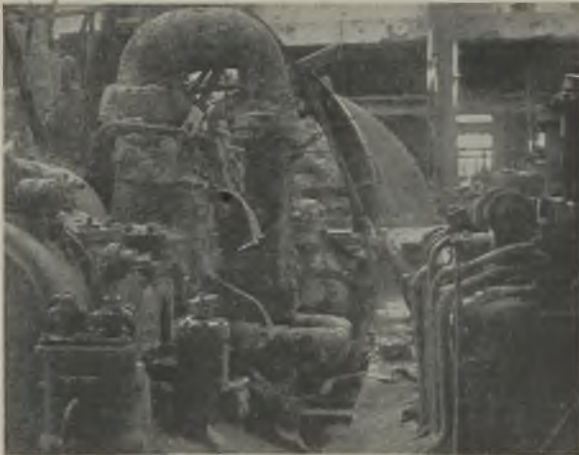
The damaged h.p. cylinder and governor gear of one of the Fulham turbines
