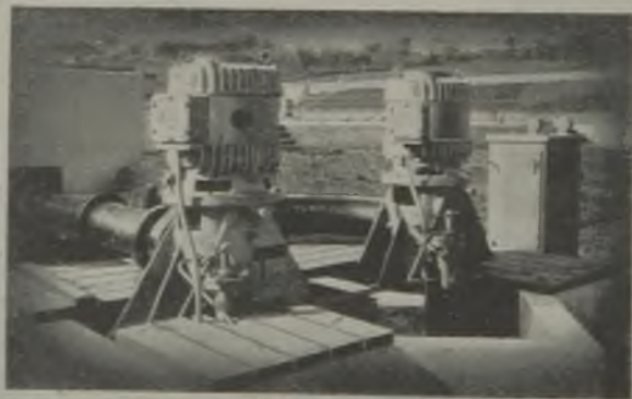
L.D.C. Weather-proof Motors, operating in the open, driving Sludge Pits.
