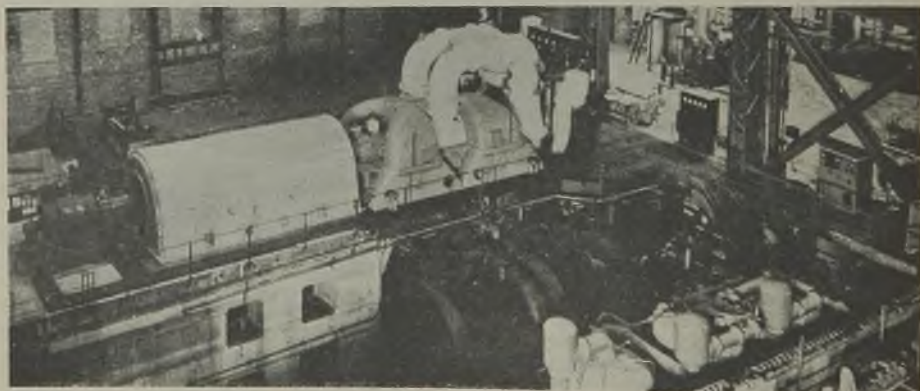
No. 1 turbo-alternator; the sea-water evaporator can be seen in the right foreground
