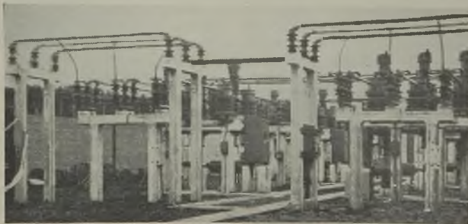
Part of the main 33-kV switchgear which is of the pneumatically-operated low-oil-content outdoor type
