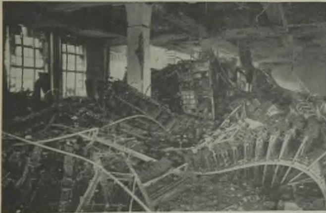
A general view of the damage at Wood Street exchange
