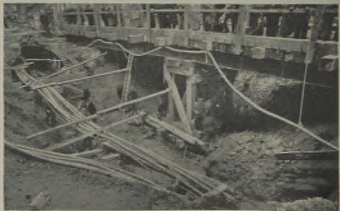
A crater in Charing Cross Road showing temporary road bridge and telephone cables being repaired
