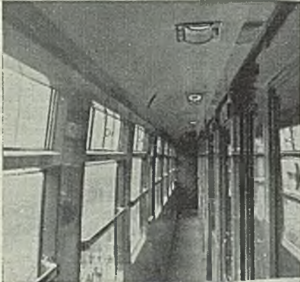
View of corridor of S. R. post-war coach, showing type of lighting installed in the compartments
