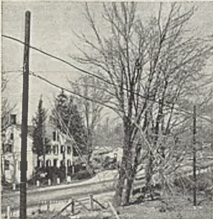
Example of aerial cable installation (seen above telephone lines) running through trees
