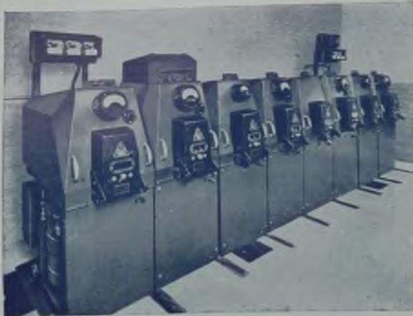
TYPICAL "IVI" METALCLAD SWITCHBOARD FOR 11 KV. 250 MVA SERVICE
