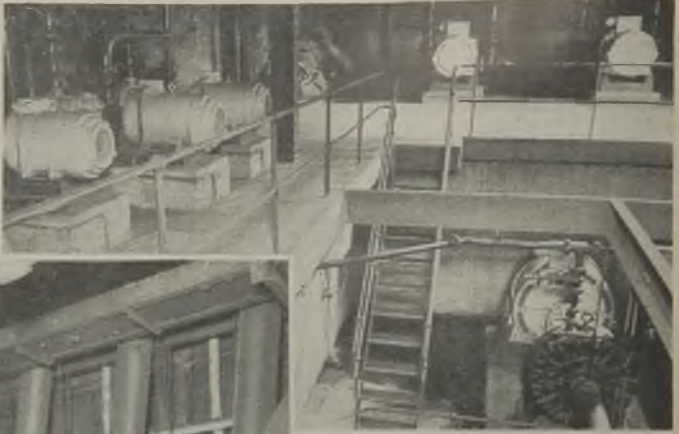
Each of the pumps in the well is in series with a pump at a lower level, and each pair of pumps lifts the ashes and water to the disposal ground up the valley; sluicing pumps are shown at floor level in the rear and sealing and quenching pumps are on the left
