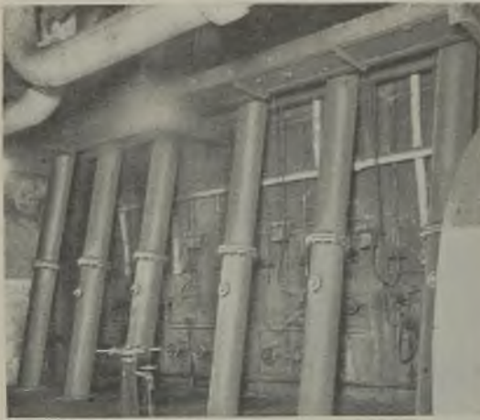
Pulverised fuel is delivered to twelve burners, via six feeder pipes, at the top of the combustion chamber because of the characteristics of the Welsh coal used
