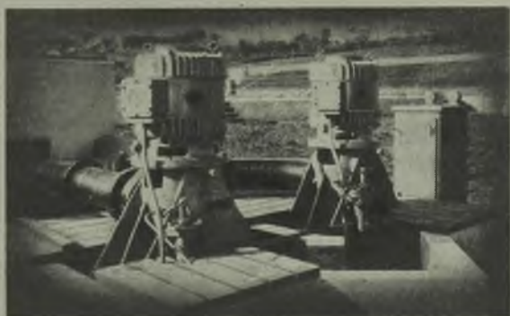
L.D.C. Weather-proof Motors, operating in the open, driving Sludge Pumps.
