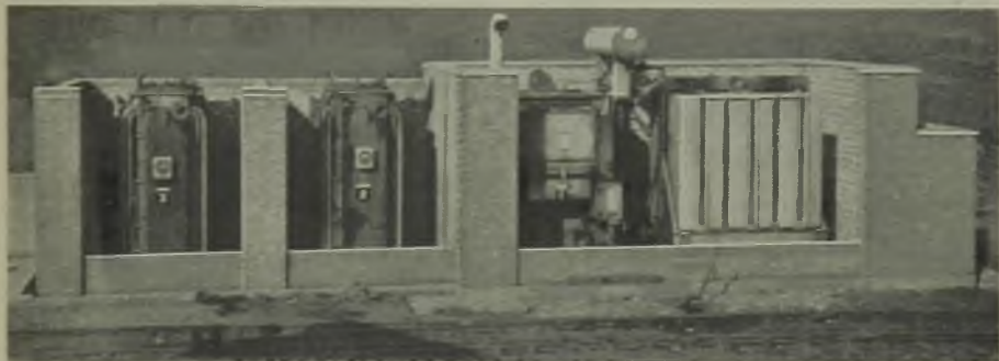
Two 5,000-kVA and one 10,000-kVA 6-6/11-kV interbus transformers supplying the new 11-kV switch-house at the power station
