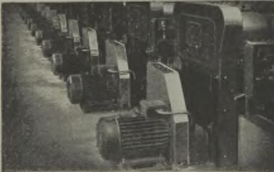
L.D.C. Totally Enclosed Fawkuhd Motors installed in a large Cotton Mill.
