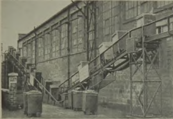
The installation may be regarded as a continuous conveyor system with the loading and unloading ends near one another outside the factory
