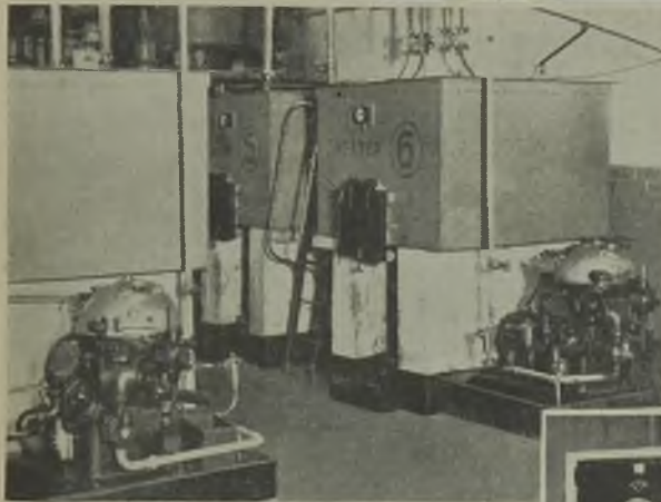
Incorporated in each of the centrifugal machines is a pump which conveys the oil to tank reservoirs; pump and centrifuge drive by the same motor
