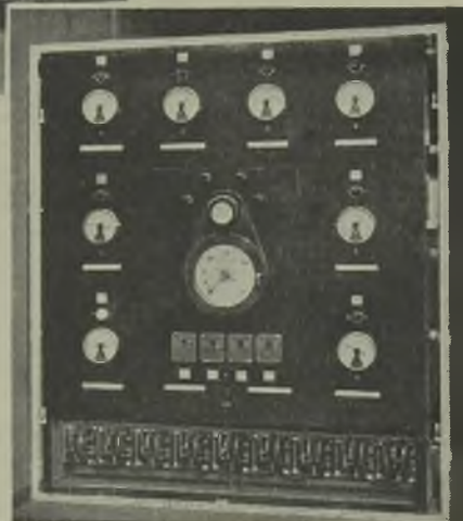
Gauges on the central control board have contacts which operate relays and, in turn, pilot lights and audible alarms
