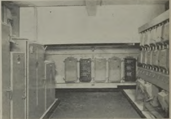
All the motors are controlled by push-buttons which operate contactor equipment in a central control distribution room; distribution equipment on right
