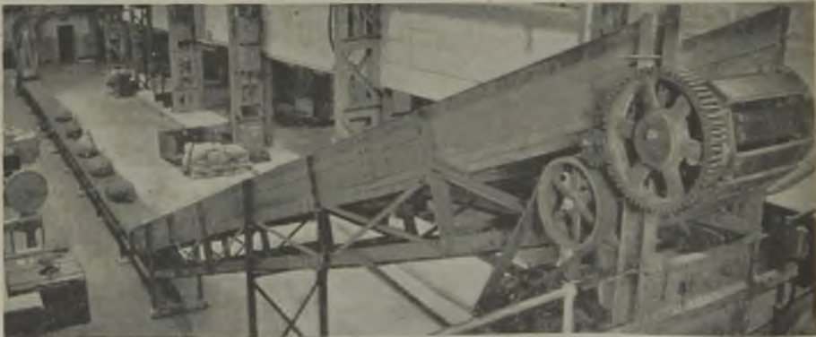
A conveyor and a chute deliver the filled bags to a straight run from which they are elevated to an unloading platform. Note conveyor drive at conveyor top on right; guard removed for photograph
