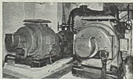
Two 275 H.P. slip-ring motors driving main shaft pumps at a colliery where the pumping plant runs 12 hours continuously every day throughout the year
