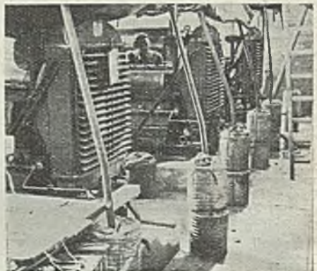
Three 15 kVA Lister Diesel generators at Wesel repeater station
