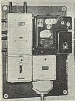
The unit installed in a 3 x 2 ft. recess with a large prepayment meter
