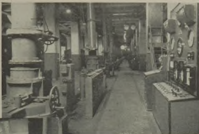
Boiler-house control equipment
