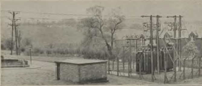
The 33-kV line is fed from a step-up substation near the Kilmarnock power station in which are installed two 5,000-kVA transformers
