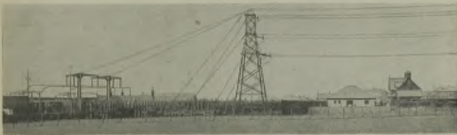
There are two sources of incoming supply in the area; one (shown) is the grid substation at Ardrossan on the coast towards the north of the area
