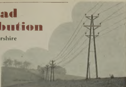
The 33-kV double-circuit line from Killmarnock to Girvan has A-pole supports of home-grown Scots fir
