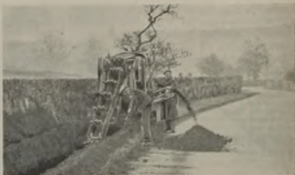
"Buckeye" digger engaged in cable laying operations for a 0.1 sq. in. 11-kV feeder from Girvan to Dailly
