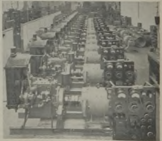
Lancashire Dynamo 6.3-kV petrol-driven alternator sets for R.A.F. mobile photographic stations
