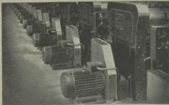
L.D.C. Totally Enclosed Fan-cooled Motors installed in a large Cotton Mill.
