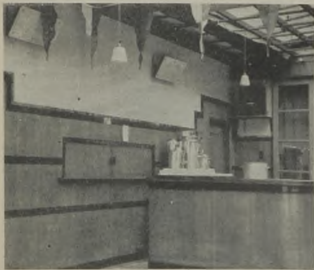
Panel heaters and cafe equipment installed in the restaurant at the Marine Hall
