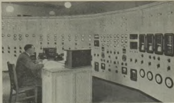
The crescent-shaped board in the control room includes panels for remote boiler control
