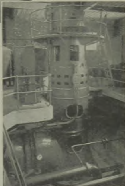
Immediately above the 3-kV AC circulating-water pump motor is a DC motor which takes over automatically on AC failure
