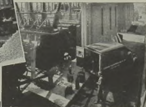
Testing a complete installation at Blackburn.
