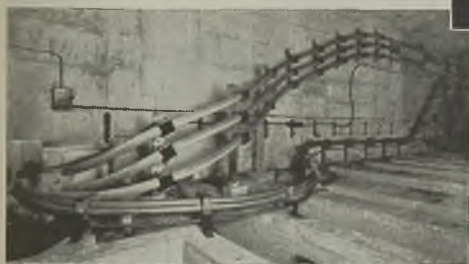
3-33 kV H.S.L. Cables, Double Lead Sheath and S.W.A. installed in Mersey Tunnel.
