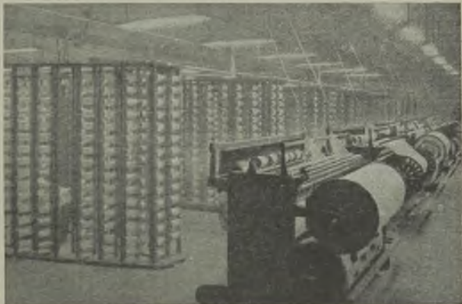
Electrically-driven warping frames at the Eclipse Mill which also has fluorescent lighting
