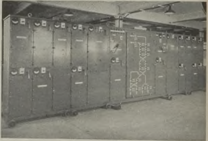
Large Brookhirst switchboard supplied to Russia
