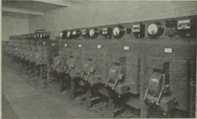
Fifteen-unit medium-voltage board controlling transformer secondaries and works cable feeders. Centre unit is a busbar coupler
