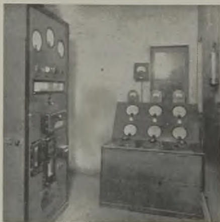
A main control panel provides for operating the air-blast circuit-breaker and the transformer tappings, and the actual furnace operations are effected from a control desk
