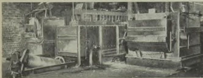
In some cases the work is brought out from the quenching medium by a worm conveyor (left). The 60-kW carburising furnace (right) has an output of 10 cwt. in 24 hours
