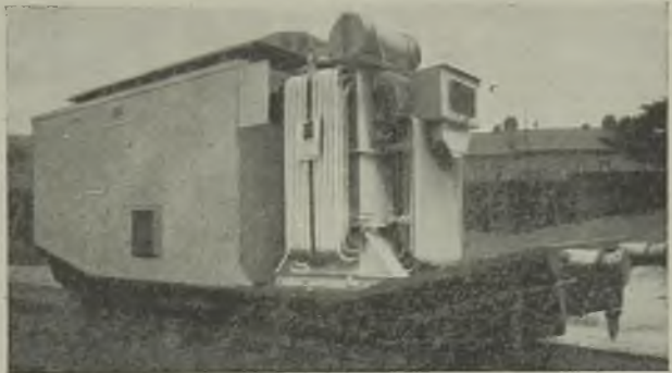
Mobile rectifier substation for railway workshop supply (1,000 kW, 500 V)
