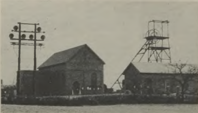
Surge absorbers have largely overcome lightning troubles. They are here seen installed on the overhead line supplying a colliery
